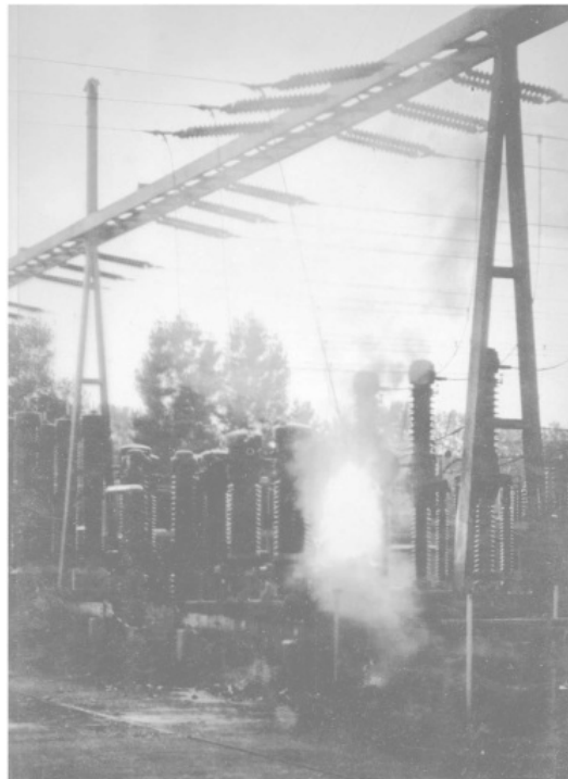
Fig. 2. Standing arc in a substation switchgear
